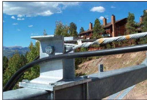
Terminus of messenger wire (only grounding between towers)
