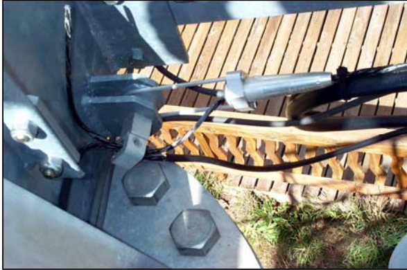
Grounding for communications cable
