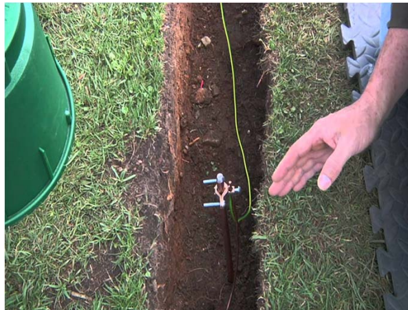
Grounding System Using Mechanical Connector with None Compliant Conductor Sizing
