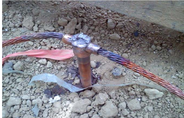
Grounding System Using Thermo-weld with Code Compliant Conductor Sizing
